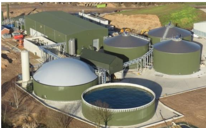
Figure 23 - UK's largest anaerobic digestion plant in Staffordshire: Business Green [56]
