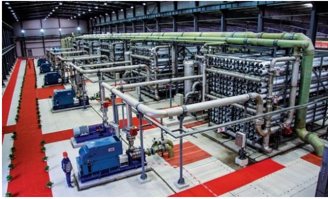
Figure 4 - Aqualyng Cangzhou Seawater Desalination Project
